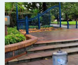
Stairs impacting access
