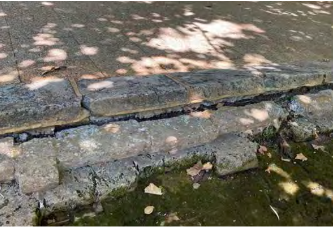
Condition of Existing Walls deteriorating
