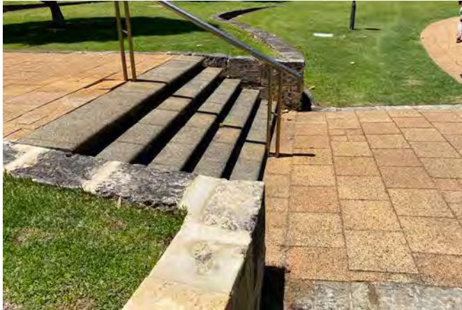
Condition of Existing Walls & paving deteriorating
