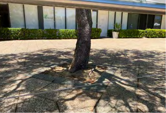
Existing trees lifting paving
