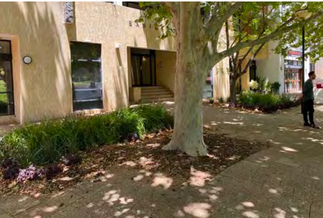
Existing trees lifting paving which creates uneven surfaces for pedestrians
