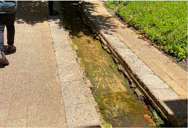
Condition of Existing water way Walls deteriorating
