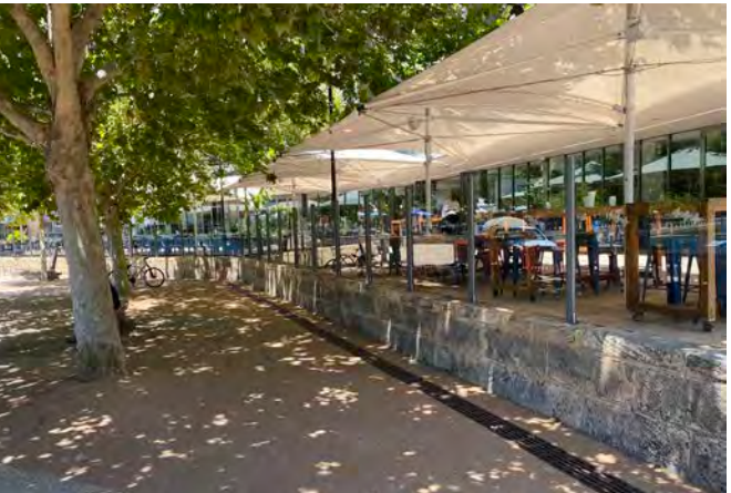
Existing trees lifting paving. Rubber softfall has been used as a temporary solution for access
