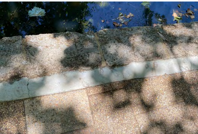
Rectification works to wall edge impacts quality & aesthetic of public realm
