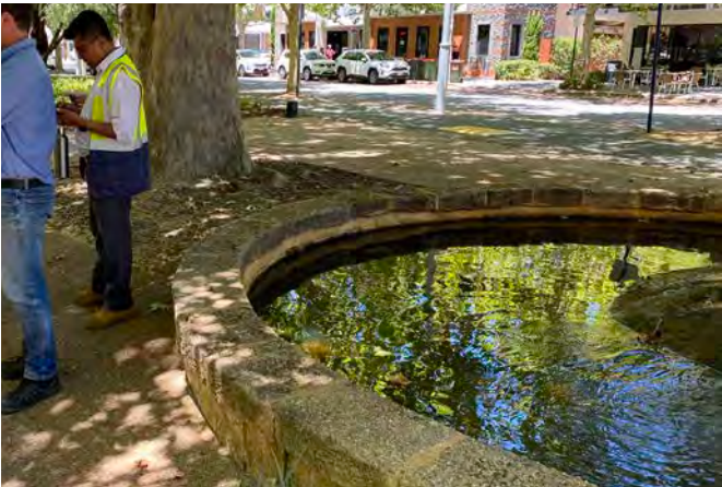
Existing trees lifting paving & impacting water feature walls
