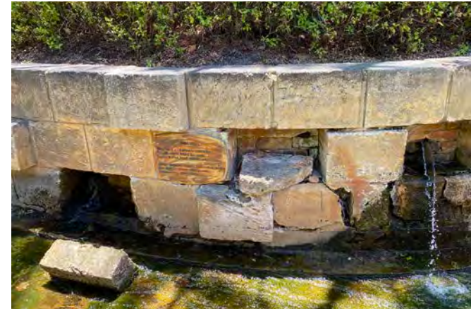
Condition of Existing Walls & water features deteriorating
