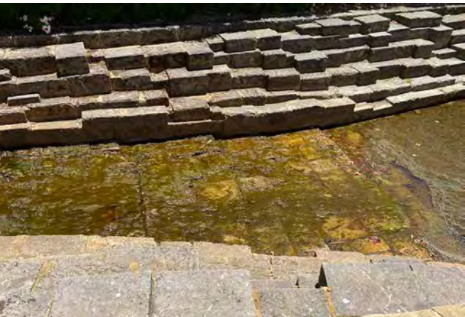
Algae build up to the water feature
