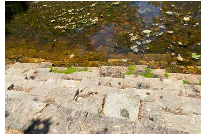
Condition of Existing Walls deteriorating impacting aesthetic & quality of public realm
