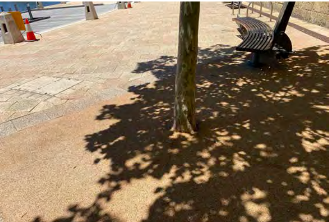
Existing trees lifting paving. Rubber softfall has been used as a solution for access
