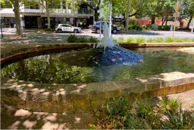
Ageing & degraded walls to water feature
